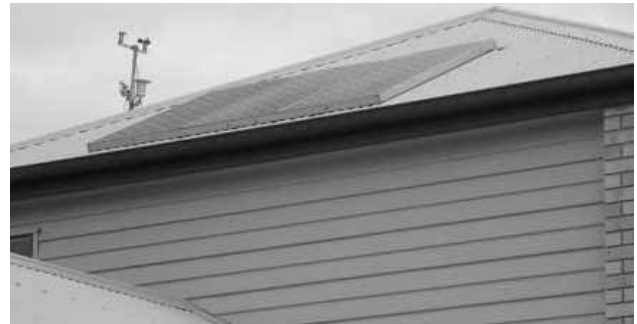
Figure 1: Solar photovoltaic panels on roof of the ecohome.
