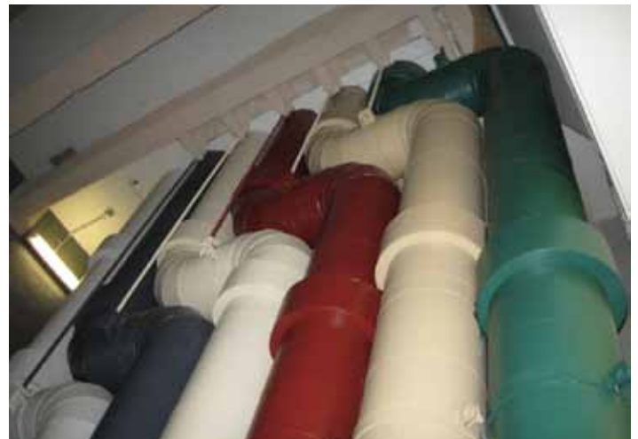
Chilled water droppers in Building 12.
